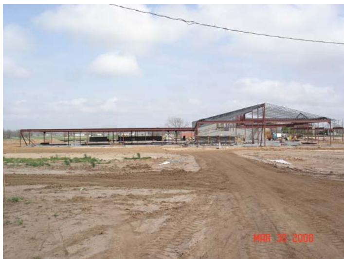
Steel columns, beams and joists. This picture was made looking to the east.
