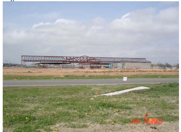
The structural steel and bar joists are being erected at the new Lexington High School. This photo was made looking north across SH-39.
