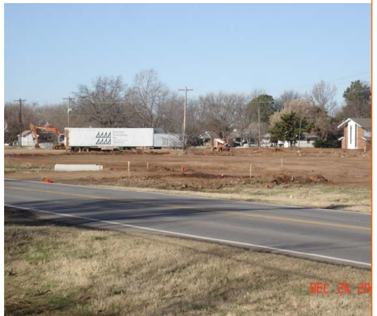
The future site of the new Lexington High School. This picture was made from across SH 39 looking northwest across the site. The Methodist Church is to the right of the picture.
